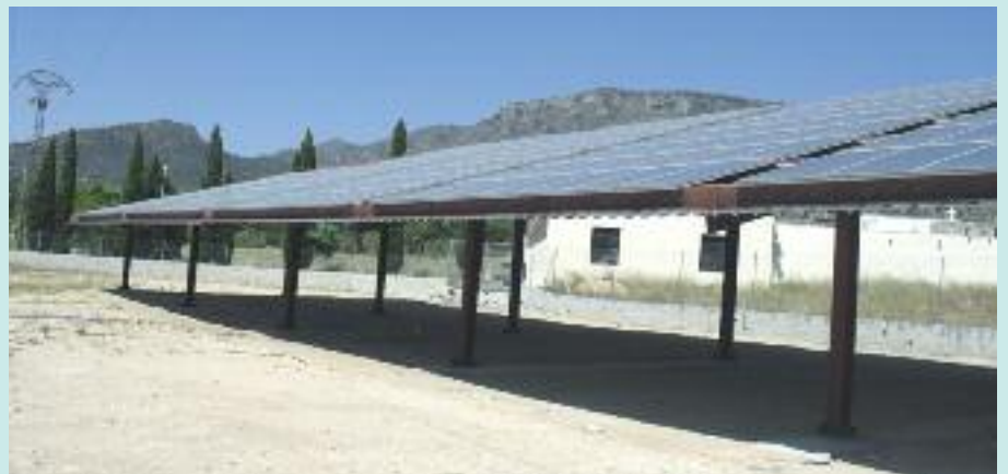
■ Solar panels will serve as a ceiling for the under cover parking of the cemetery
